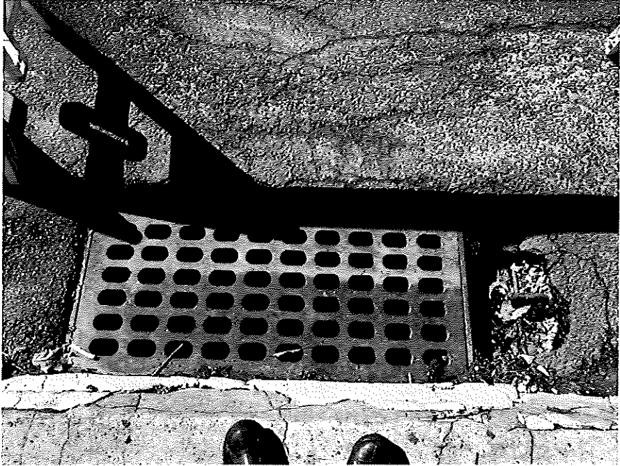
Photograph 1. Hole at Upstream Inlet, Note Visible Rebar
