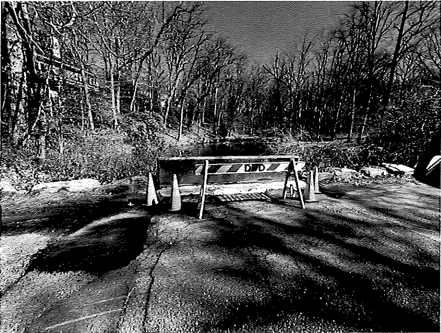
Photograph 4. Restricted Area by Demarest DPW, Note Sediment Accumulation and Settlement of Approaches
